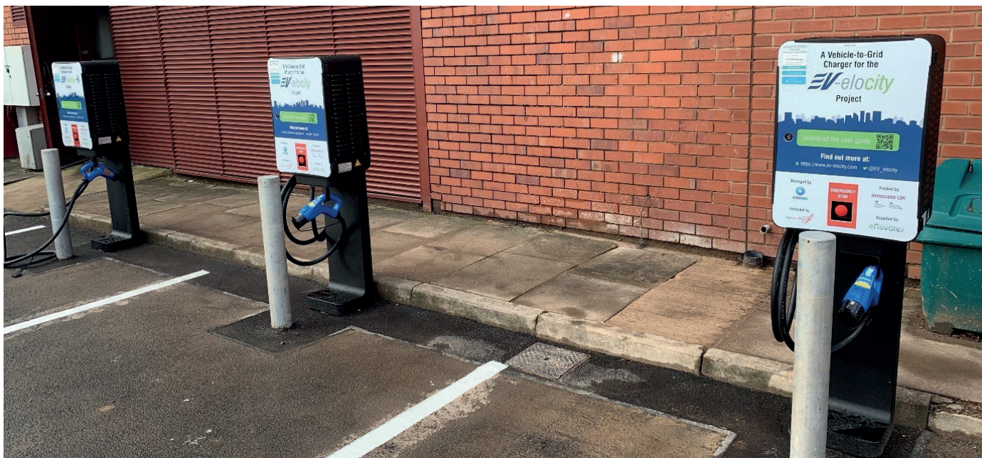
Figure 25: S04 – Charger points at the Boiler House, University of Warwick.
